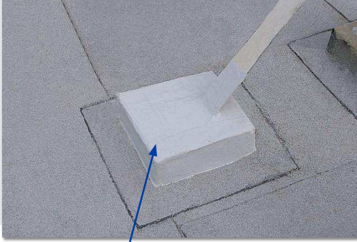
⚠ Failed Sealant Pocket
